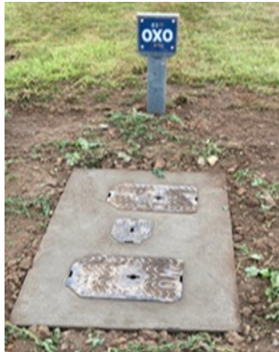
Reduce, Recycle & Re-use: • Recycled crushed stone access track • Recycled plastic valve & hydrant chambers
